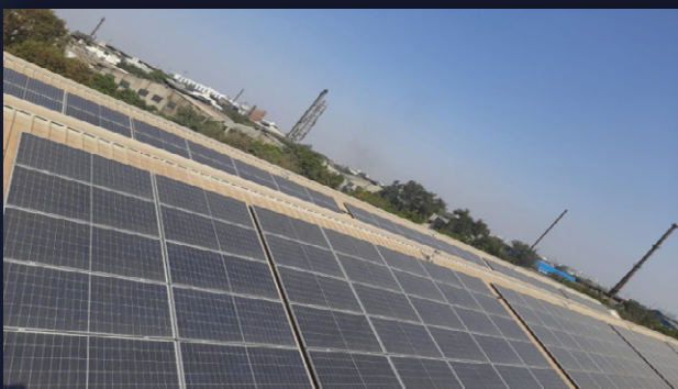
2.5 MW JTEKT India Limited, Gurgaon & Bawal
