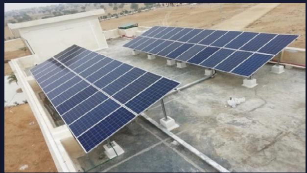
100kW, Sports Academy, churu, Rajasthan
